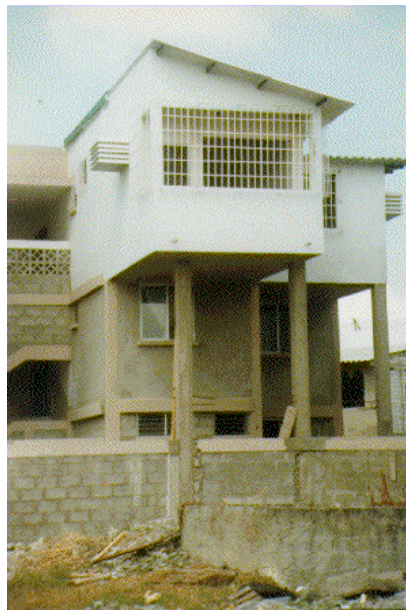
A type of structure with a high seismic risk are those condominiums built by BEV in Sauces IX, in which extensions have been built without any structural design and technical supervision. This building was expanded, been converted into a vulnerable structure due to a bad construction practice.
