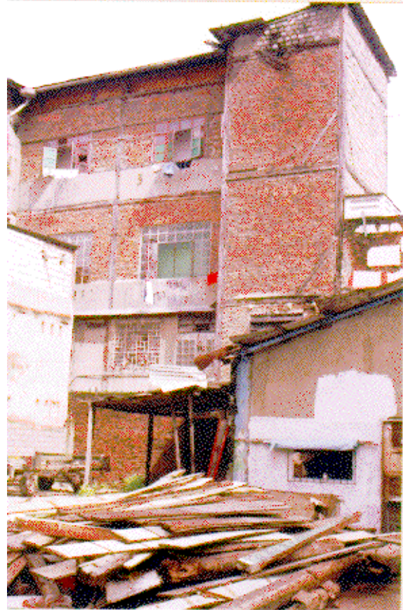
This building made of a wood structure and brick walls, is a kind of structure that can suffer severe damage during an earthquake of intensity M.M.=VIII.
